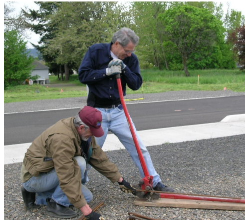
Bend it! Phil Aird and John Hocken work at bending an iron reinforcement rod for the foundation.
